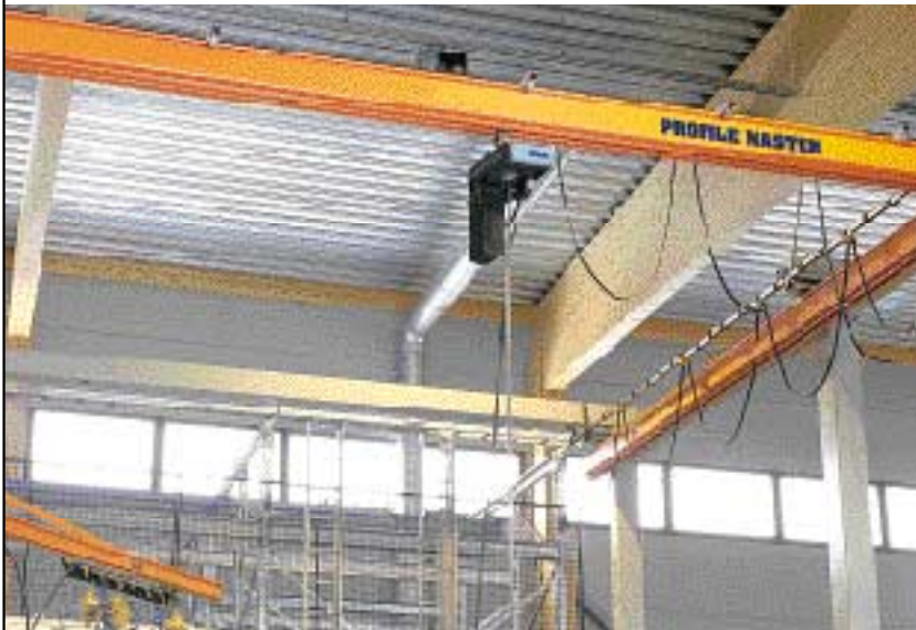
Example of ProfileMaster installation in a ware house
